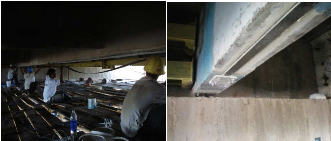
Fig 7 Pre-stressing in process and the finished laminate with anchor plates at end.
