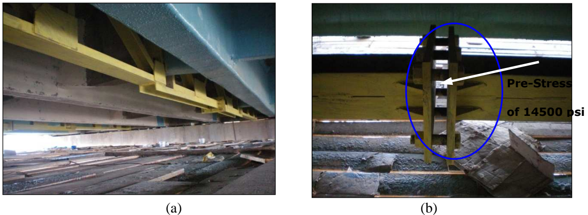
Fig. 5 (a) Connection of Truss over Diaphragm Beam and (b) Pre-stressing Mechanism in Truss During Installation of Steel Truss System
